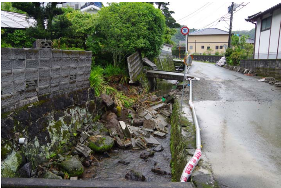
Branching fault in the Mashiki town
